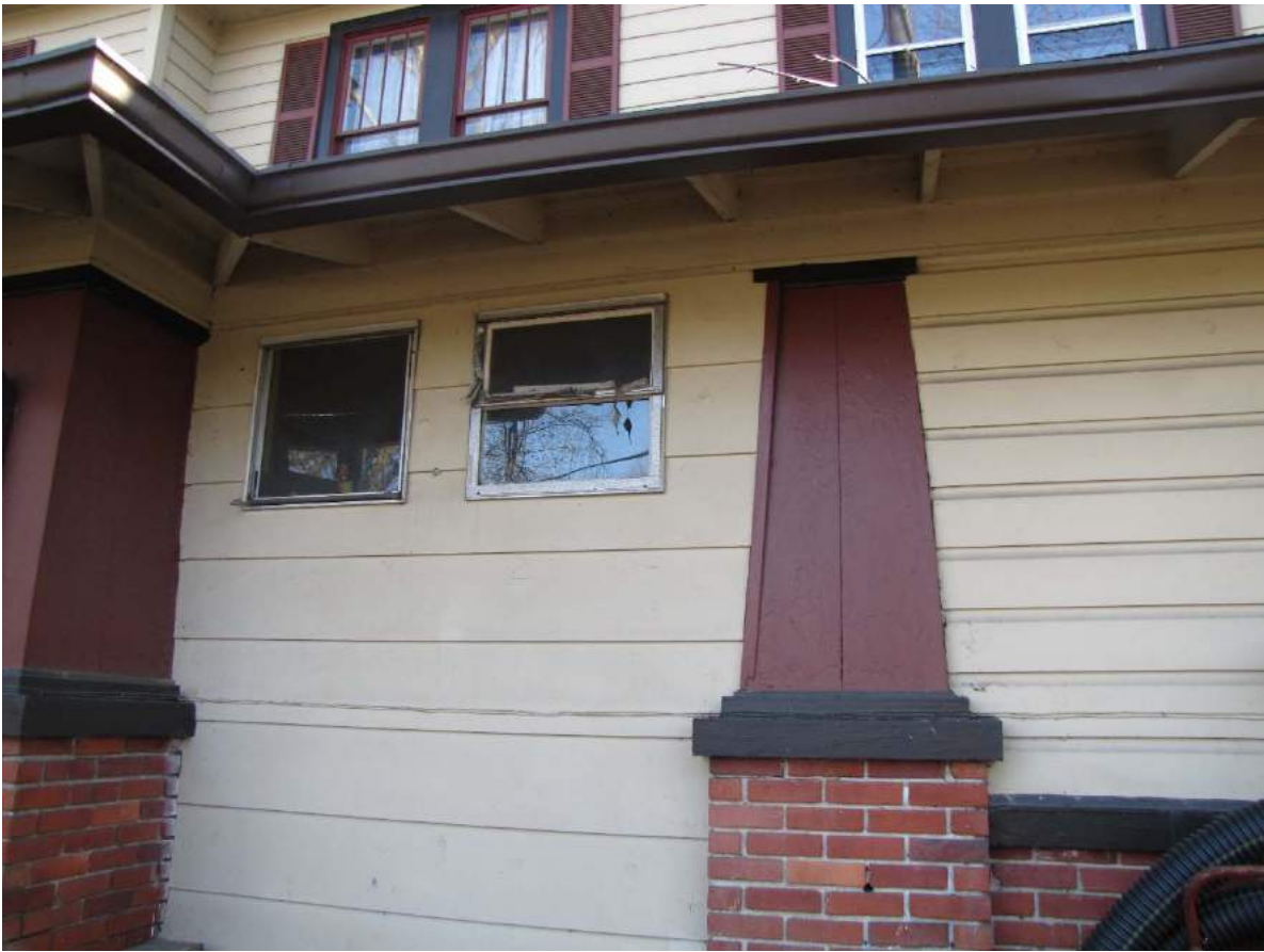
Poplar Terrace House, north elevation, view to the south, detail of infill entrance area
